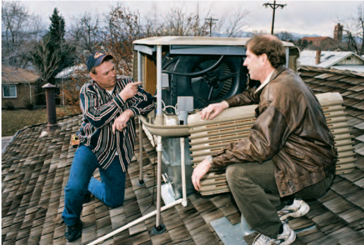
Evaporative or “swamp” coolers can be an efficient alternative when done properly.
