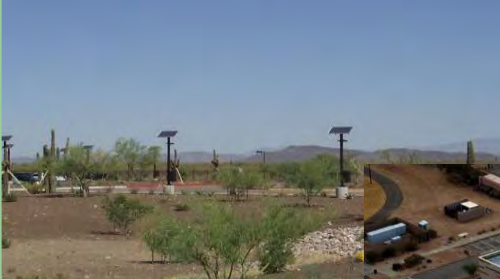
Parking lot lighting
