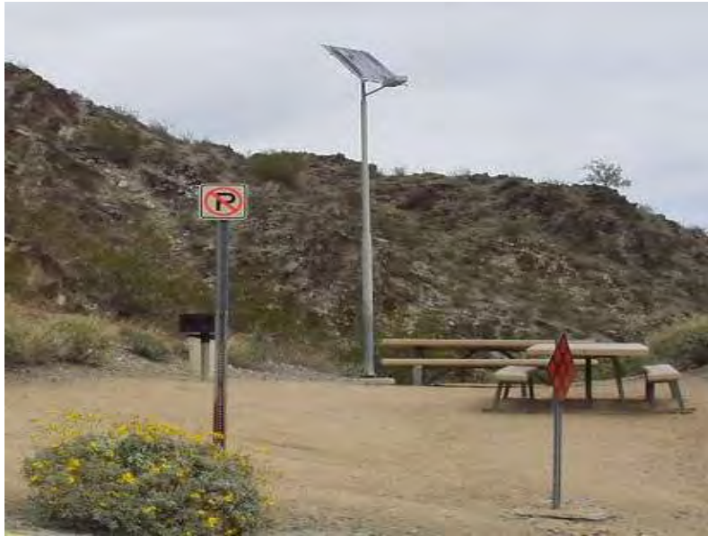
Park Security Lighting
