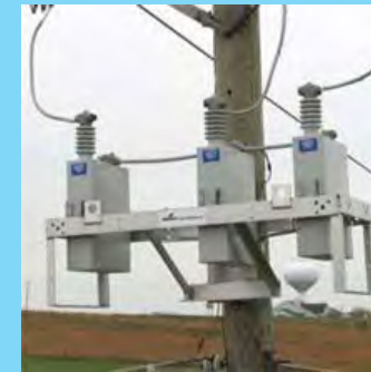
Fixed / Switched Cap Banks
